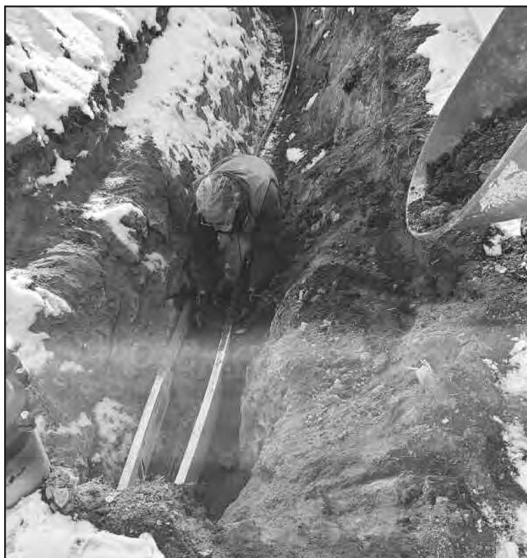
Ken Spoor working on the pipes for the new well. Ken has spent many manual labor hours working on this project for Pleasant Park Grange.
