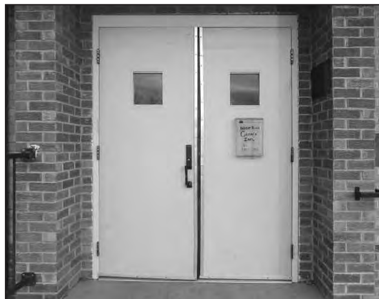
Wheat Ridge Grange hall improvements coming in January 2021 ... the front entrance will be getting new entry doors ...
